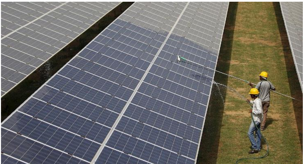
Figure 8 – Example of cleaning of PV modules
