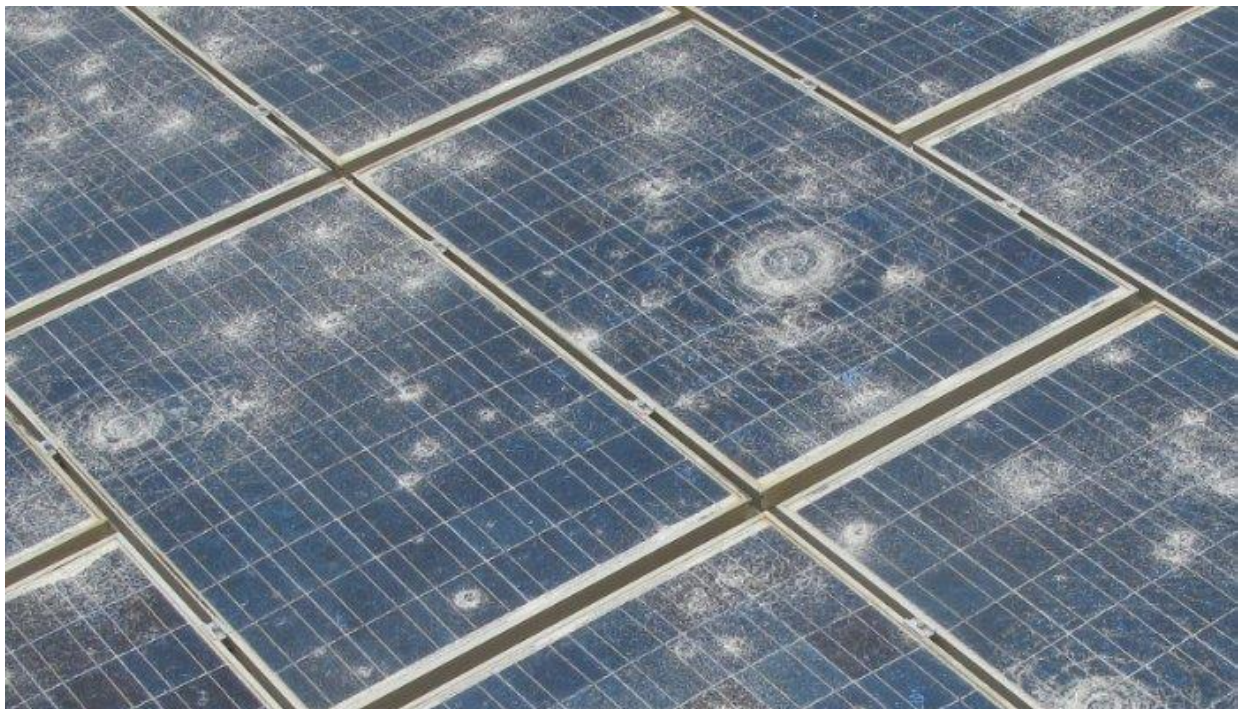
Figure 7 – Examples of hail damage on PV modules
