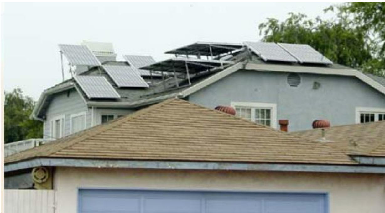
Figure 21 – Example of a poor installation on a rooftop
