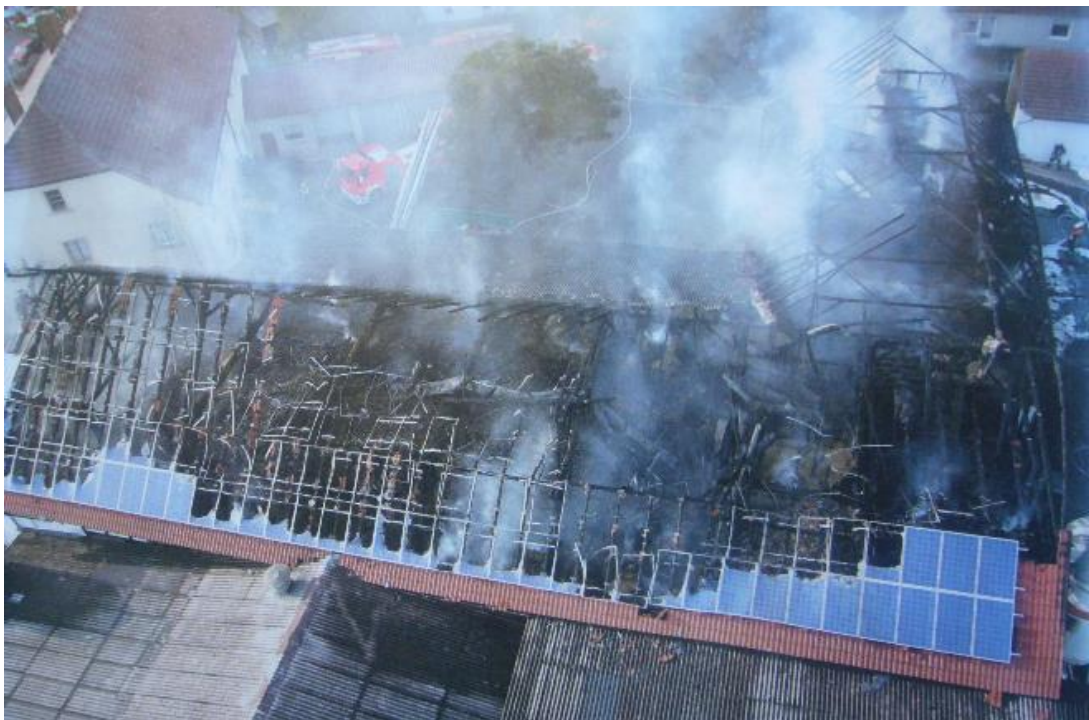
Figure 6 – Example of fire originated in a house with a PV system on the rooftop
