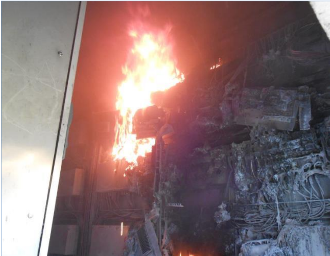
Figure 8 – Example of combiner boxes burning despite fighting operations, because they are still fed by the PV array
