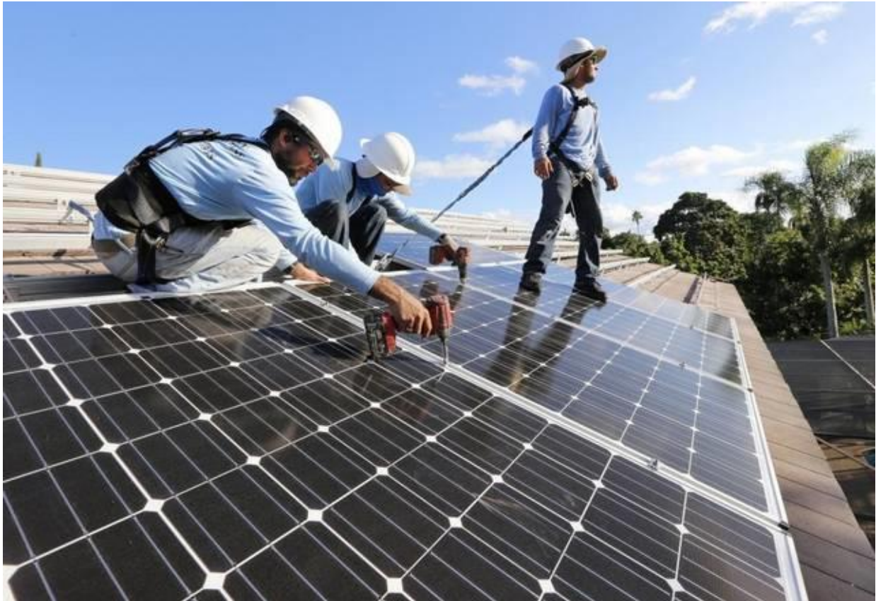
Figure 3 – Example of installation of a PV system in presence of several risks
