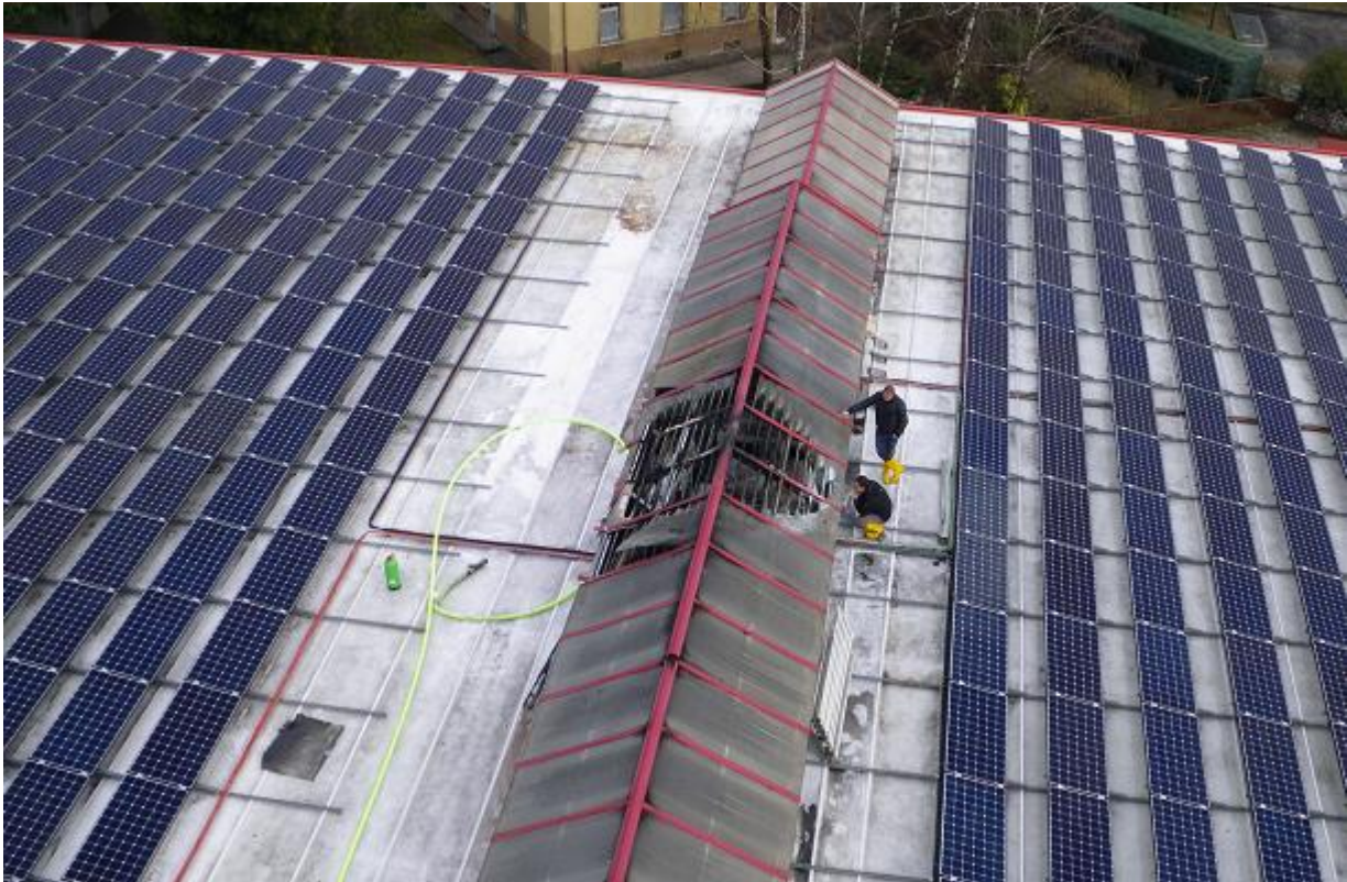
Figure 7 – Example of effects of a fire in a PV system originated in combiner boxes
